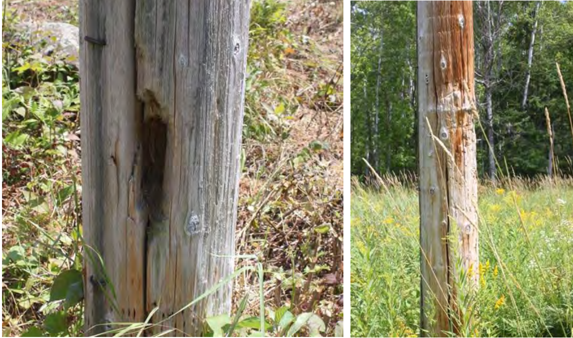
Figure 13. Poles damaged by bears and general wear and tear.
