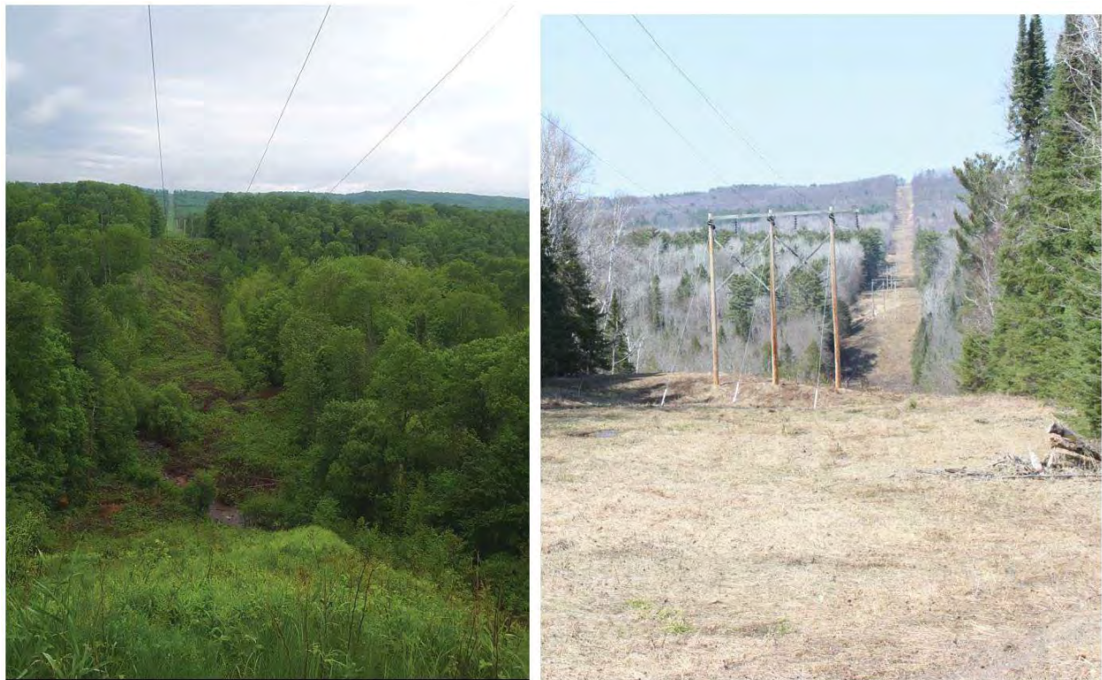
Figure 4. Pictures of long spans on existing line with 3-pole structures.
