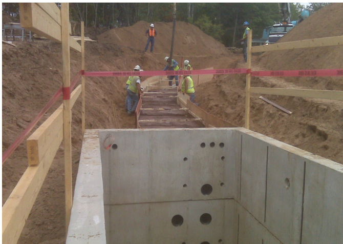
Crews work on an underground duct bank extending from a typical 8'x 8'x24' vault
